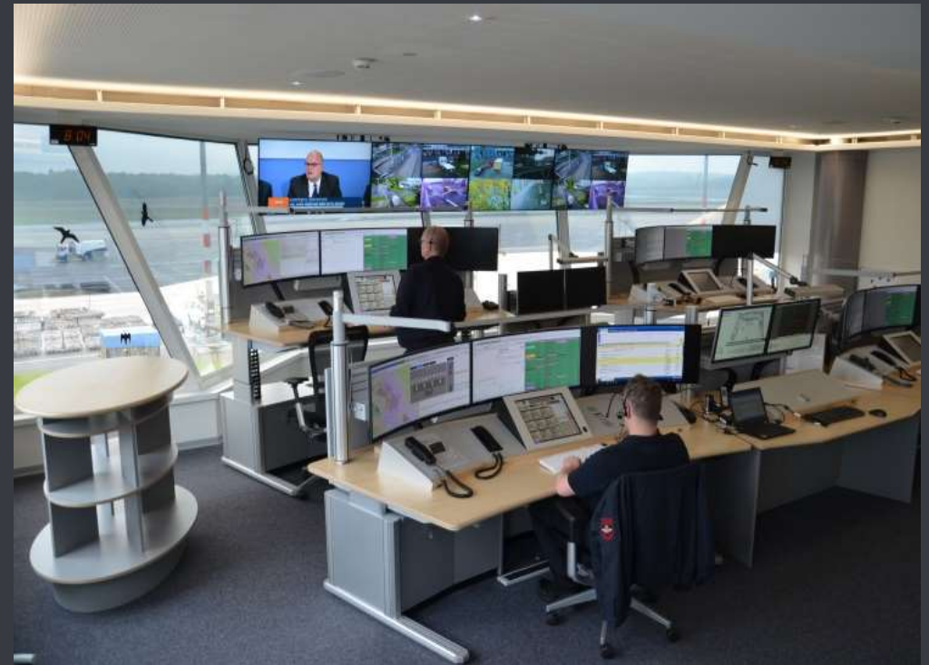
Emergency control center / Airport Köln-Bonn (CGN)
