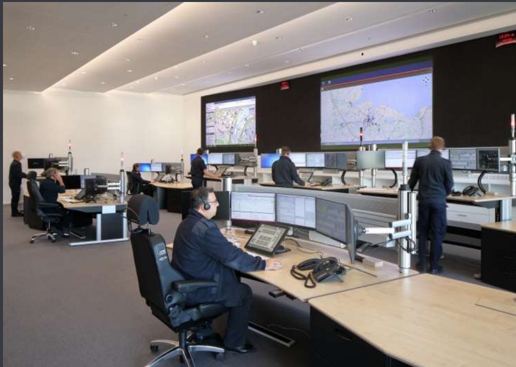
Regional emergency control center / Firedepartment Kiel
