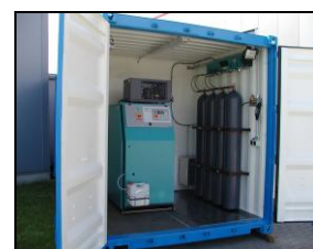
Compressor container - interior view
